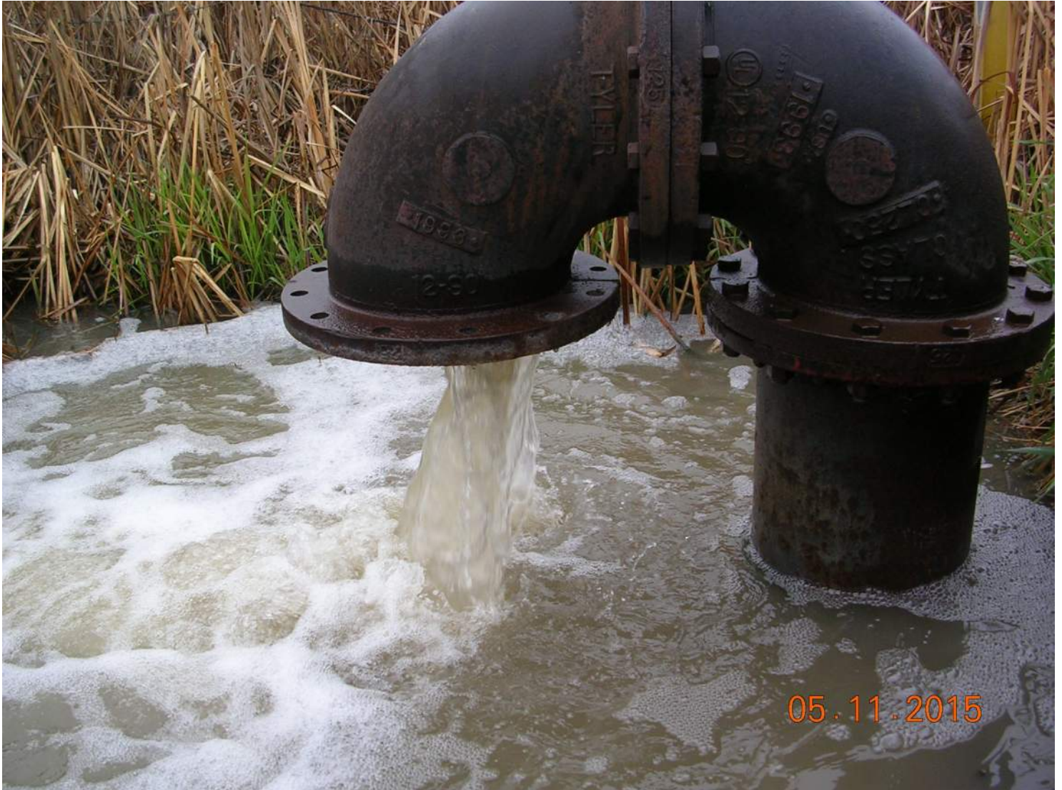
Storm sewer lift station discharge pipe
